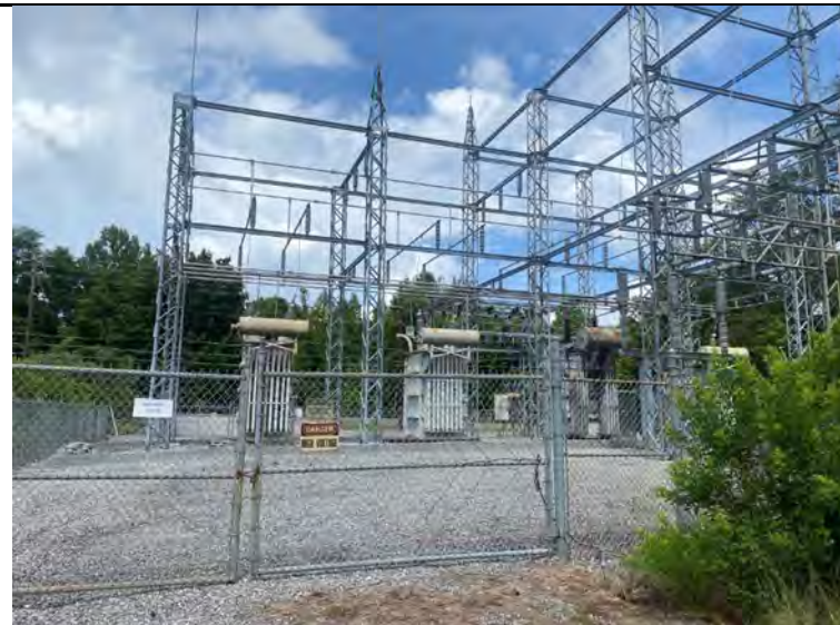
Photograph 12 – Bad Creek Substation (Facing East)
