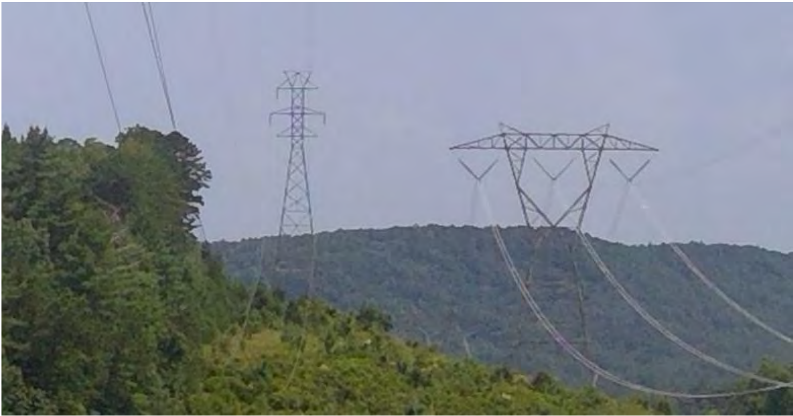
Figure 5-2. Steel lattice, Jocassee Set-up SW-Bad Creek 100-kV (left side of ROW) and the Jocassee Tie to Bad Creek Hydro 525-kV (right side of ROW)
