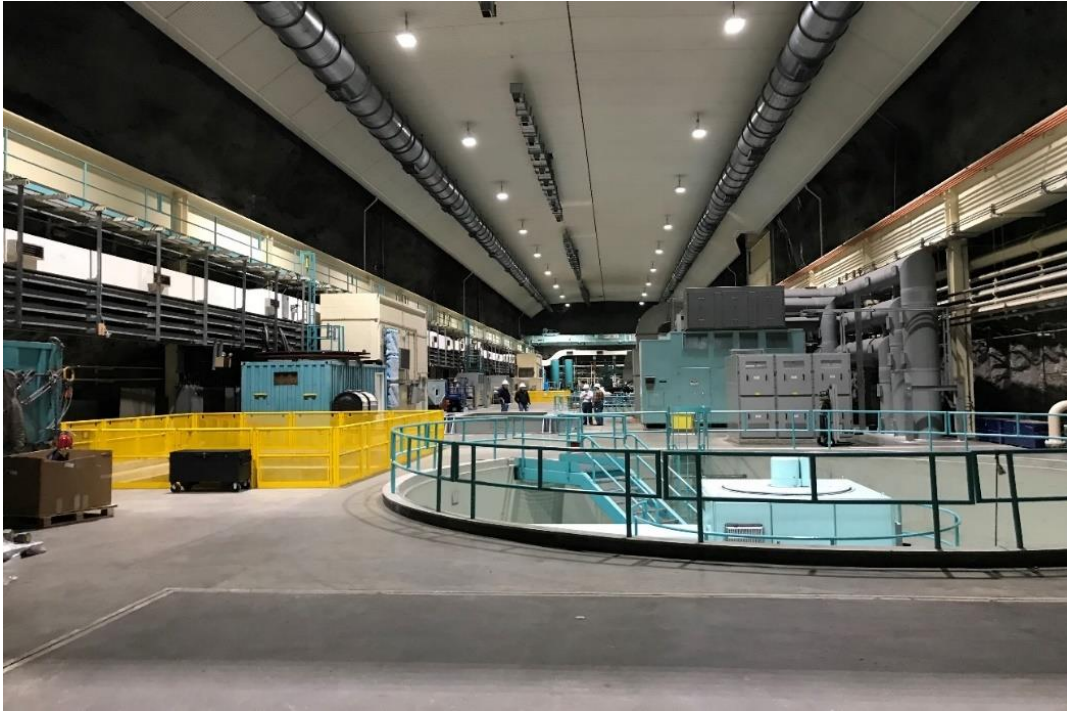
Figure 5.4-10. Bad Creek Project Operating Deck
