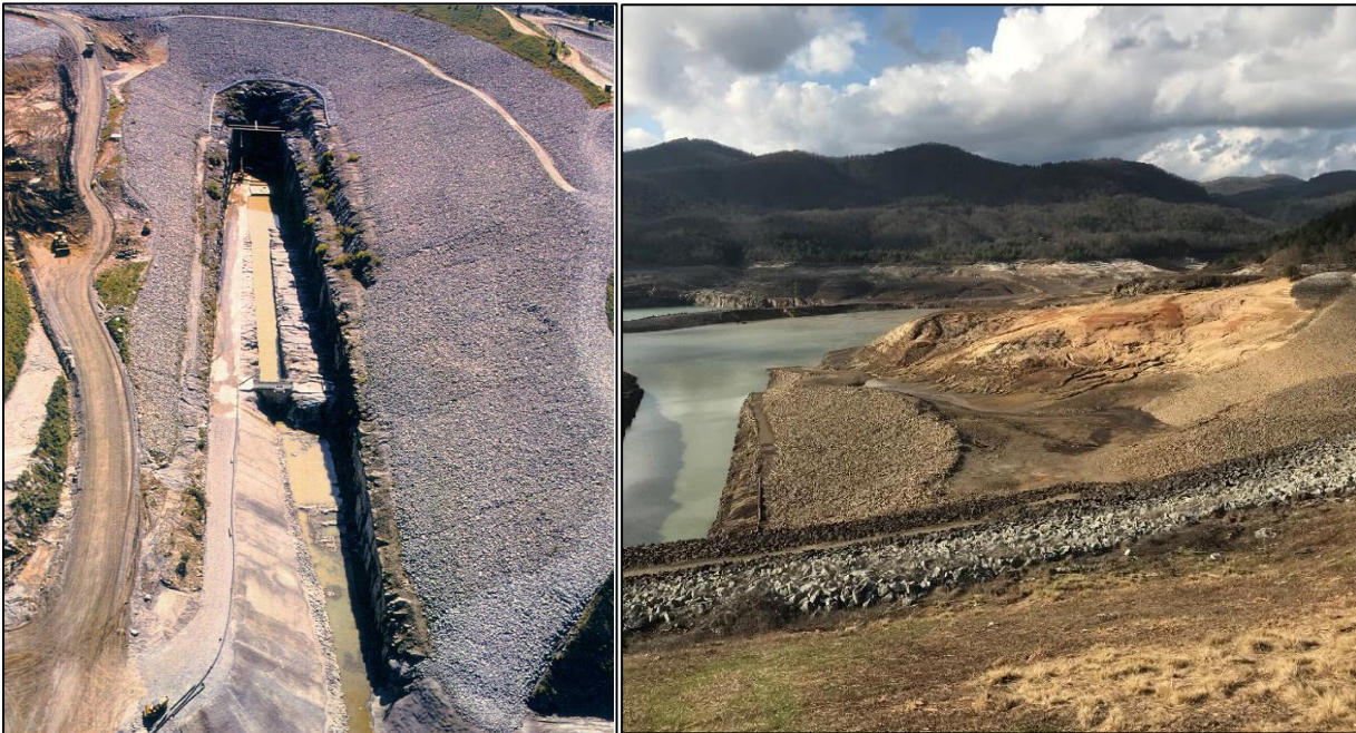
Figure 5.4-4. Upper Reservoir Intake Channel; (left) Prior to Initial Reservoir Fill and (right) Under Full Reservoir Drawdown Condition
