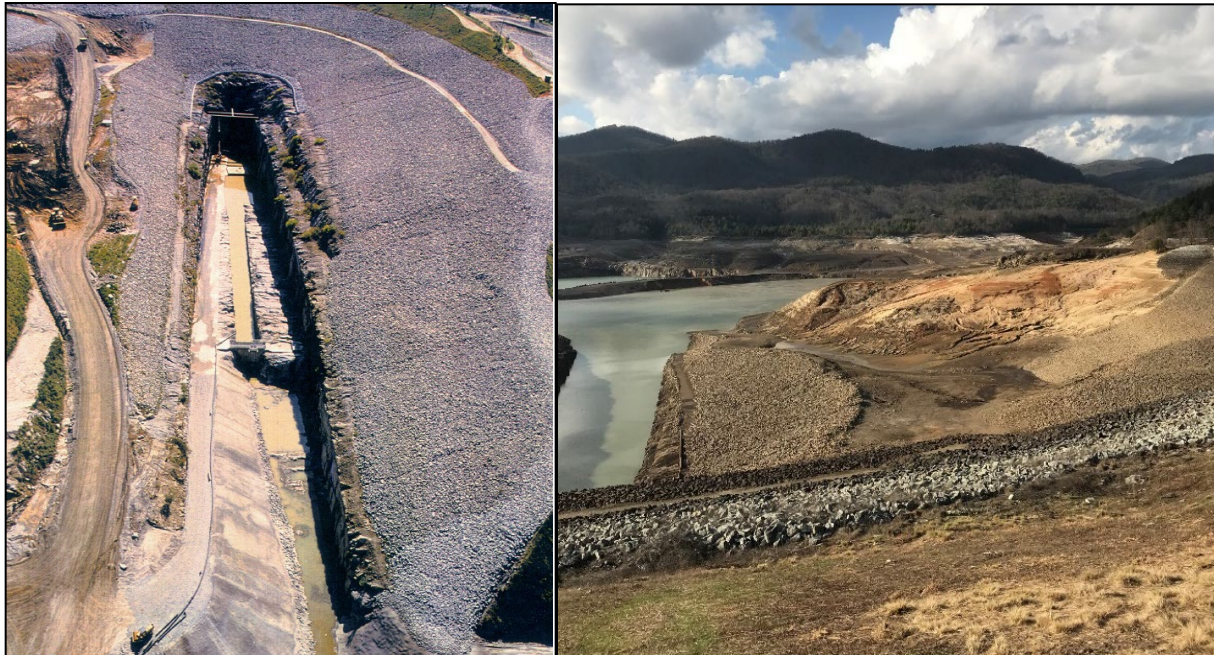
Figure A-5. Upper Reservoir Intake Channel; (left) Prior to Initial Reservoir Fill and (right) Under Full Reservoir Drawdown Condition
